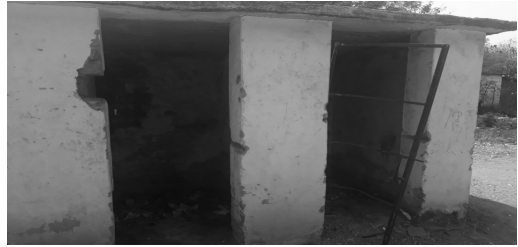
Figure 2. Toilets in Dilapidated Condition
